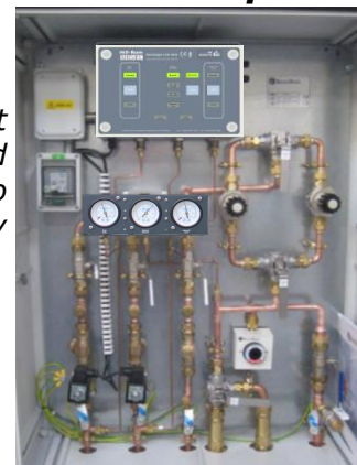
View inside panel
